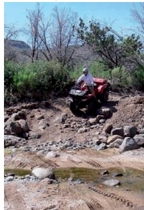
Washed out section of road.
